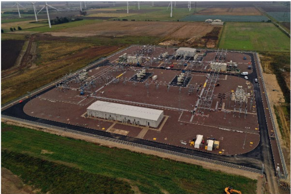
Plate 5.29 Onshore substation (image courtesy of RWE Renewables)
