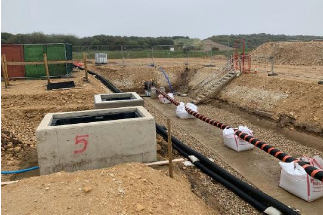
Plate 5.17 Example transition joint bay including the concrete link boxes – the tops of which are the only structures that are visible above ground once reinstatement is complete (image courtesy of RWE Renewables)
