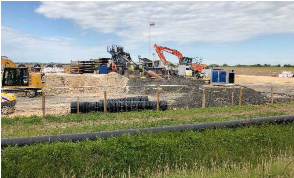
Plate 5.16 Example of an HDD drill rig at landfall – the cable duct is closest in the foreground (image courtesy of RWE Renewables)
