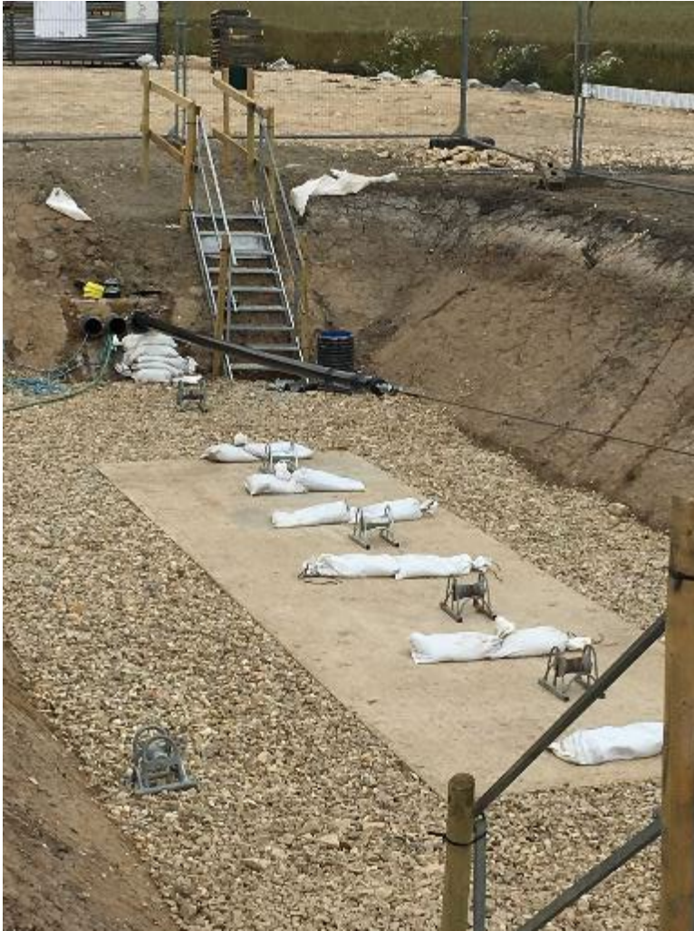
Plate 5.25 Example jointing bay with cable pulled through (image courtesy of RWE Renewables)
