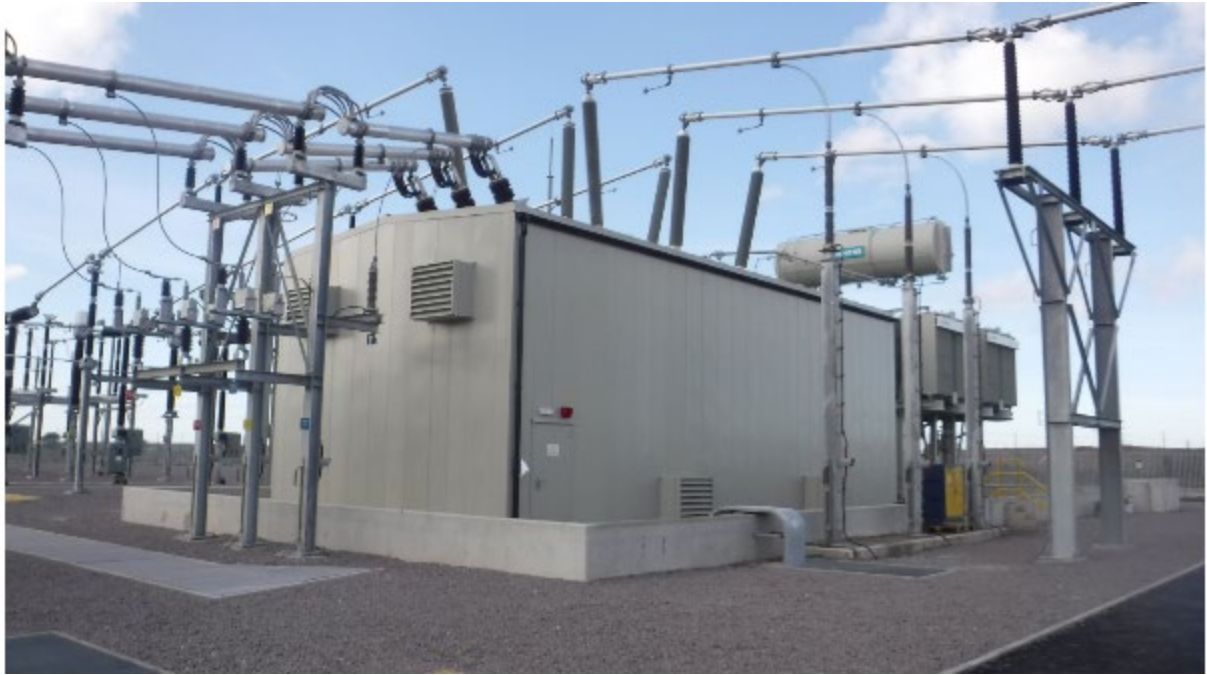
Plate 5.28 Transformer with noise enclosure (image courtesy of RWE Renewables)
