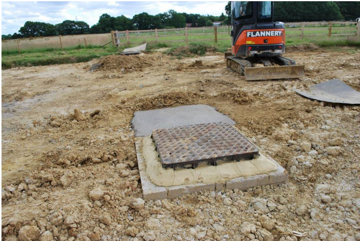
Plate 5.26 Example link box following reinstatement (image courtesy of RWE Renewables)
